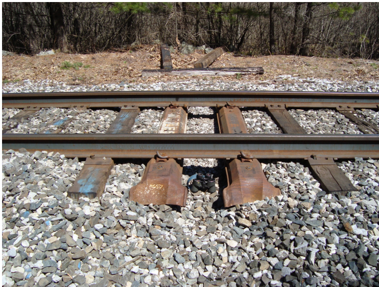
Figure 6: Underpass installed on railroad track in southeastern location. Binoculars placed in crossing to give scale. (Photo credit: S. Parren)
