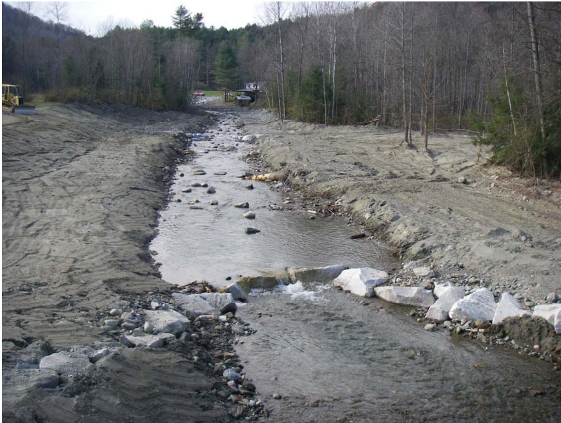
Figure 12. Camp Brook (Bethel) following instream channel restoration. Stream channel dimensions were improved but limited availability of materials precluded the restoration of aquatic habitat diversity and complexity.
