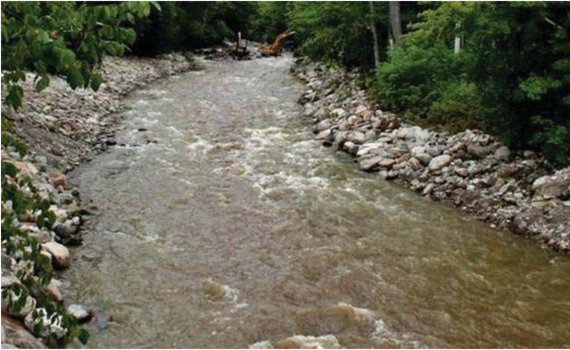
Figure 8. The Middlebury River (Middlebury) showing excavators in the process of removing coarse material from the streambed and creating berms along the streambank.
