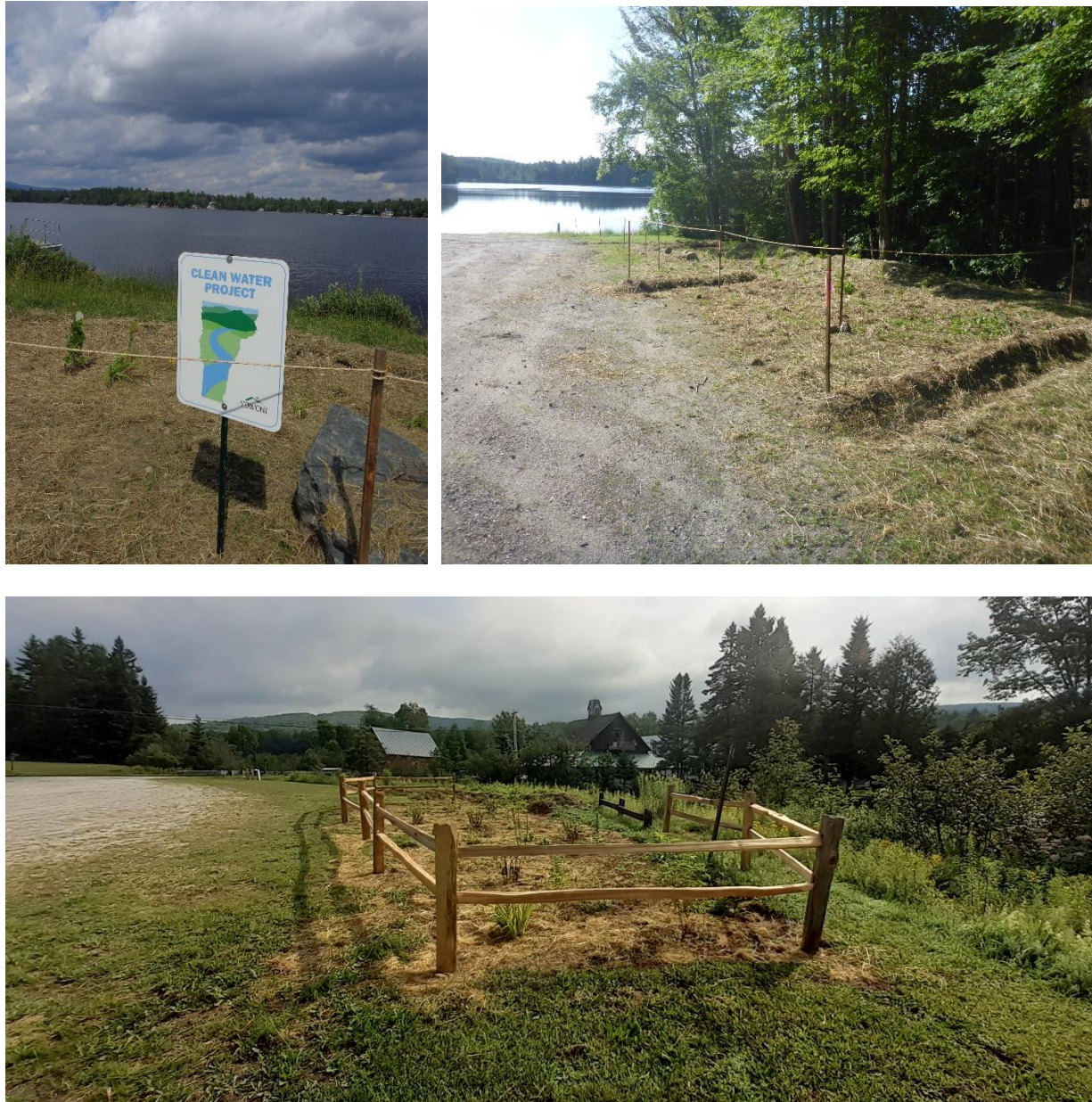
Figure 2. Three stormwater improvement projects were completed during the summer 2019, where vegetated retention areas were created to capture, filter, and infiltrate run-off from parking areas. Prior to these improvements, stormwater would run directly from the parking areas into the lake or to a ditch, which directed water into the lake. From top left clockwise: Island Pond, Spectacle Pond, and Seymour Lake.
